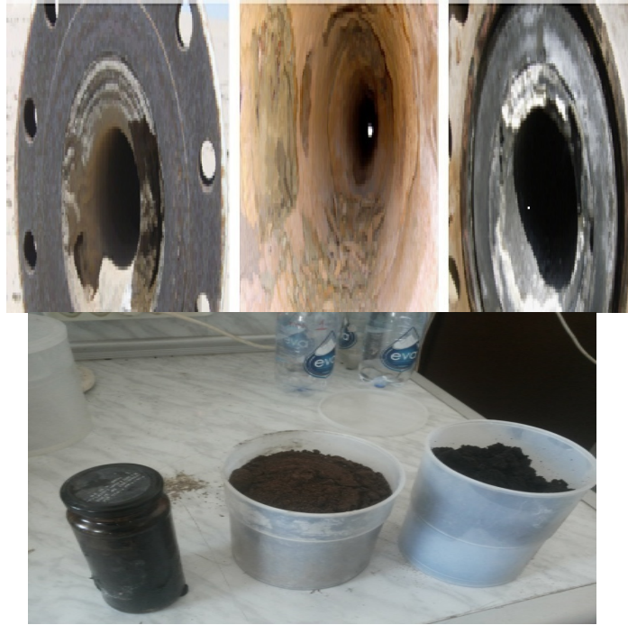
Figure (3) Scales inside the pipes
